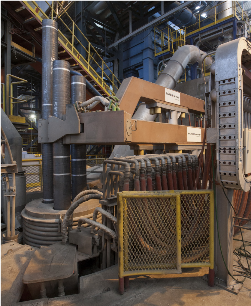
Twin-ladle furnace built by SMS group.
