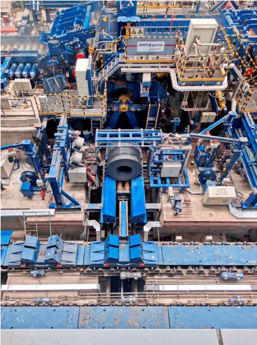
One of three down coilers at the new high-performance hot strip mill of HBIS Laoting.
