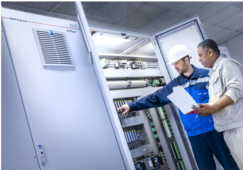
X-Pact ® automation cabinet at Al Ezz Dekheila Steel Company (EZDK).
